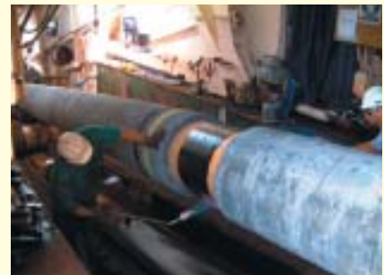
A Canusa-CPS wraparound sleeve is installed to protect the girth weld on concrete coated pipe.
