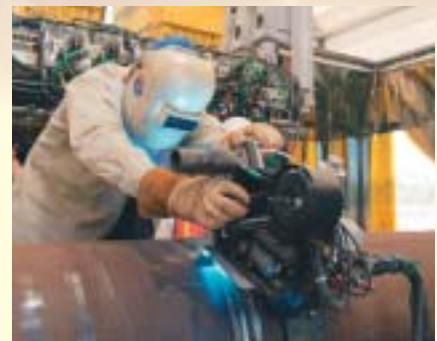
Specialized welding equipment utilized by Bredero Shaw to weld offshore flow lines and risers.
