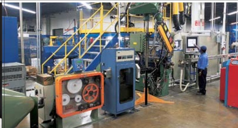
NEW, COMPUTER-CONTROLLED EXTRUSION LINE INSTALLED AT THE SHAWFLEX WIRE AND CABLE FACILITY IN TORONTO, ONTARIO.
